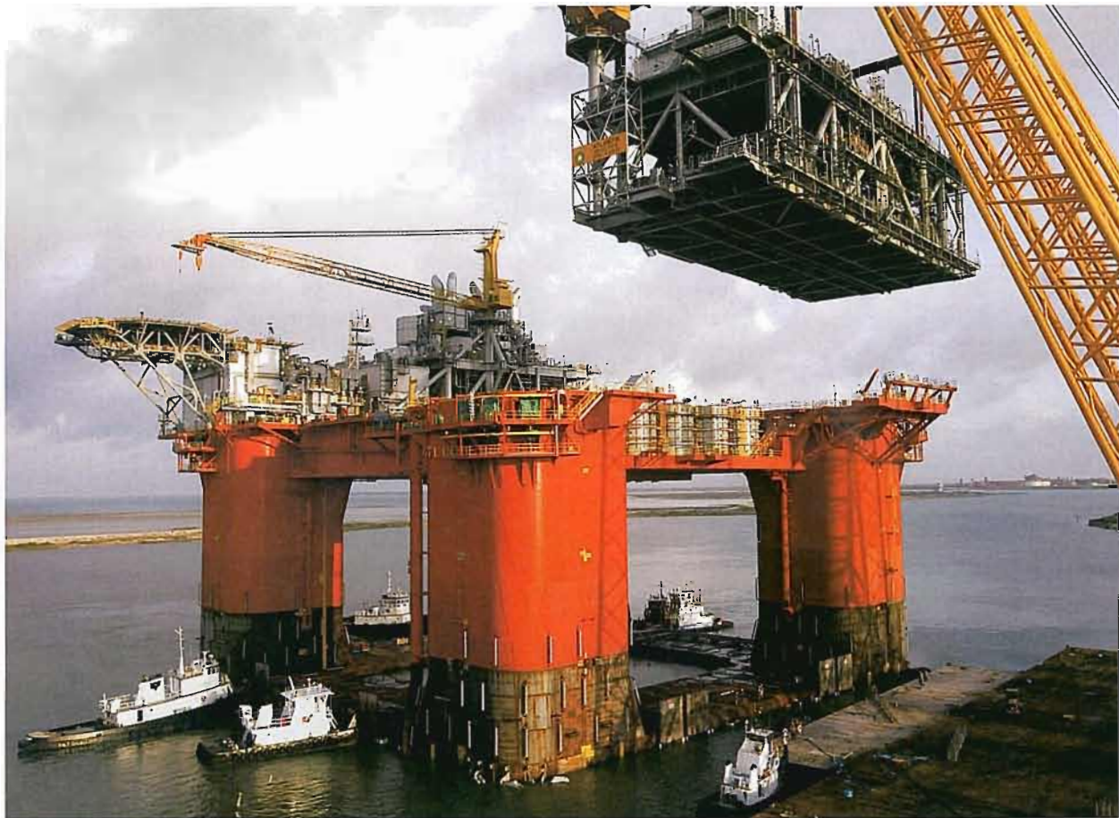
Atlantis, at 46,856 metric tons, is being assembled in the Coastal Bend region and will be the deepest moored oil platform in the world.
