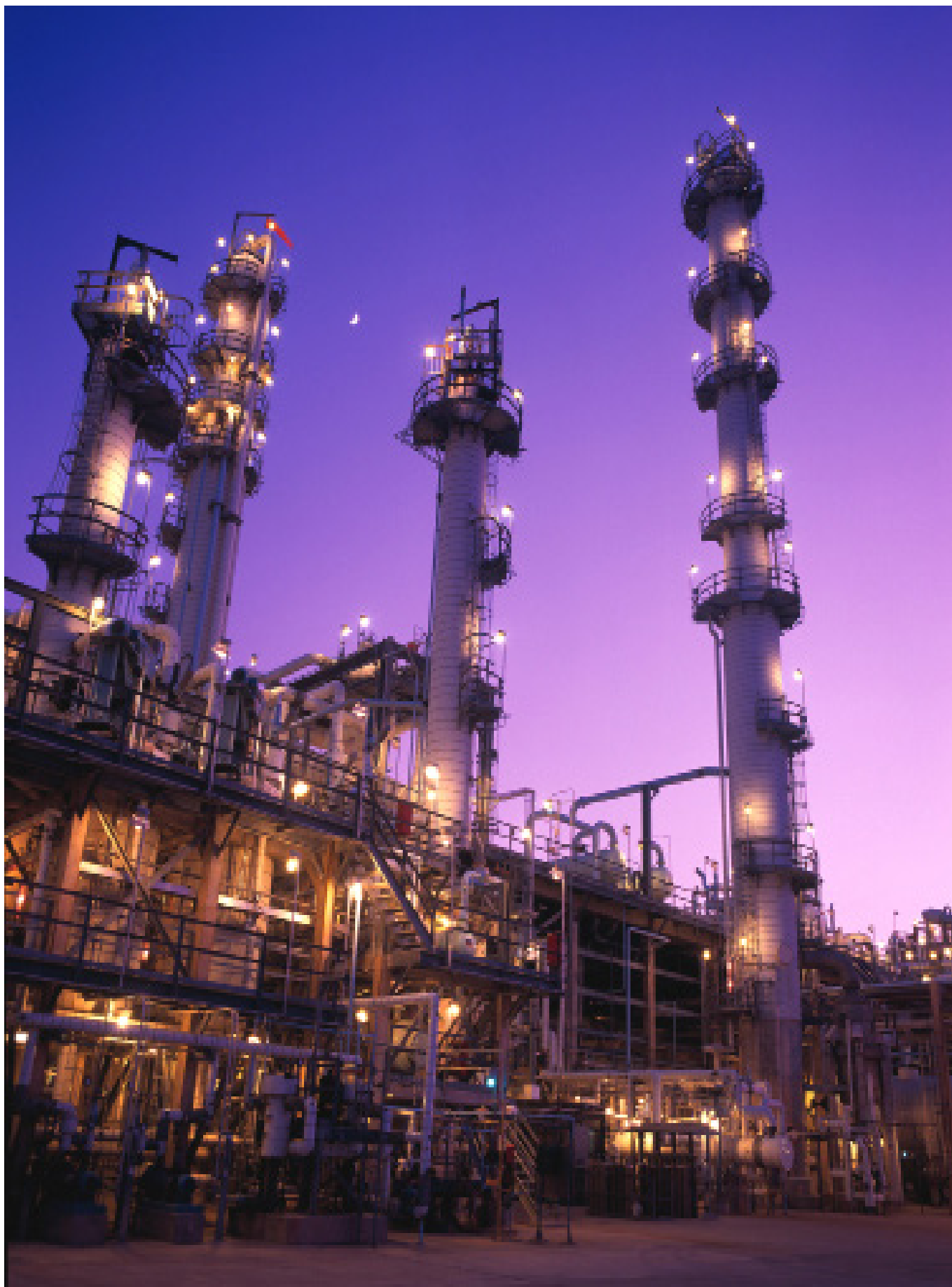
Refinery Photo Courtesy of Atex Delvalle
